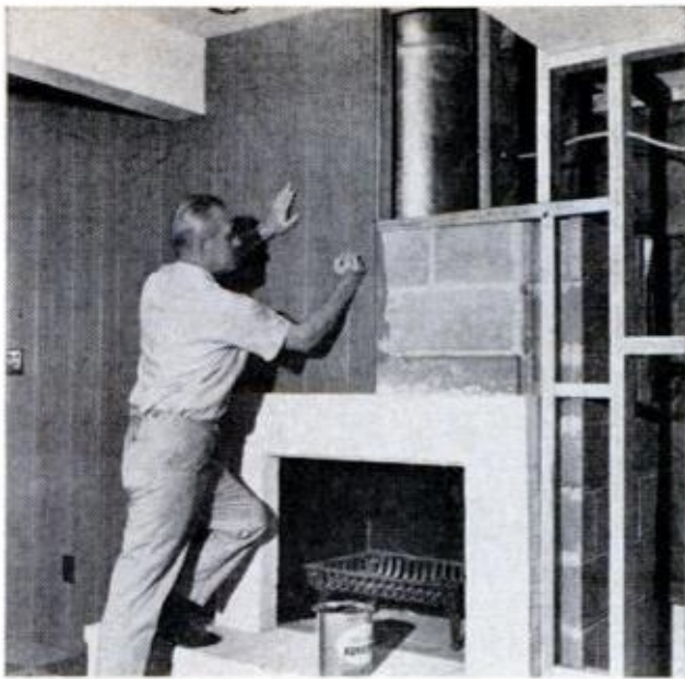
TAPPING PANEL WITH FIST after you have it in position assures a good bond. Work quickly as the mastic sets up fairly fast, with little time for shifting
