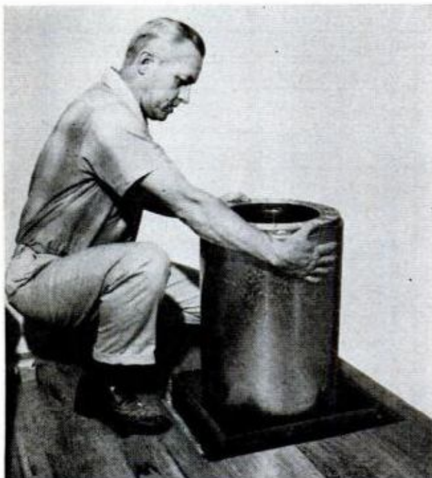
TWISTING MOTION locks pipe sections together as they're stacked. Here pipe passes through firestop
