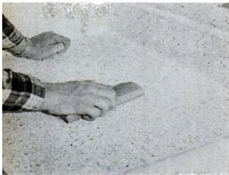
SAND LIGHTLY and then vacuum to remove all dust and loose chips. Check and repair any bare sections
