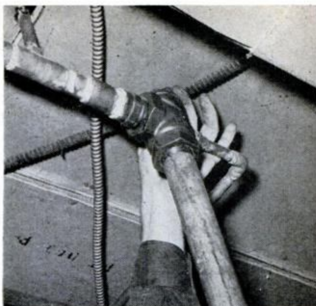
FLOW VALVE , usually hidden in a corner, can be opened to feed hot water through system by gravity
