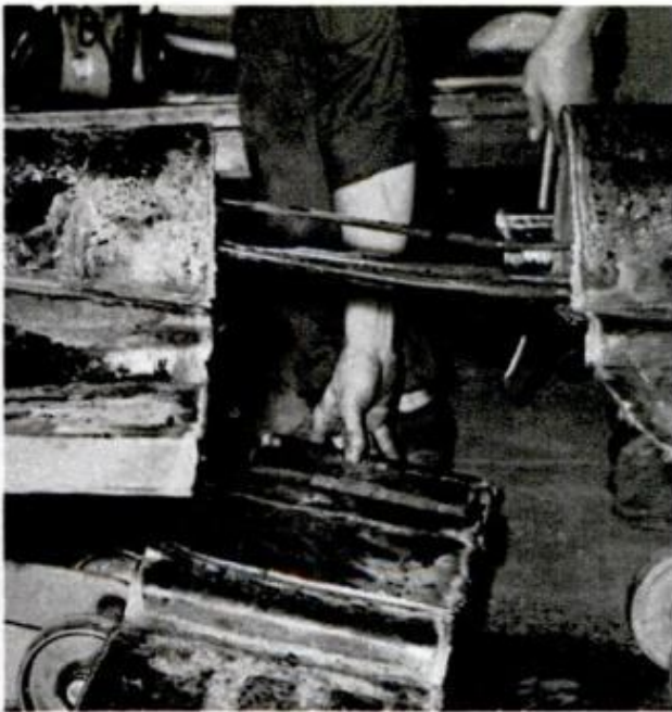
WHEN MAKING CUTS to remove 10-in. section, be careful that control cables in tunnel aren't damaged
