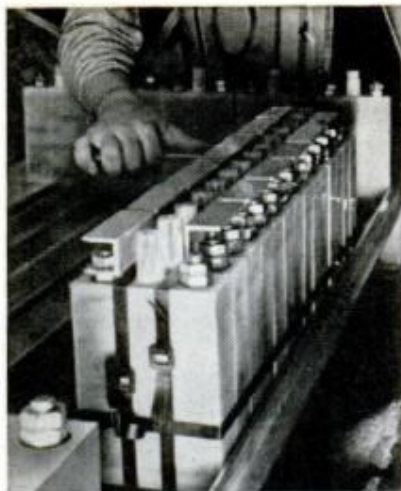
NICKEL-CADMIUM cells, rated 75 ampere-hours each, are installed
