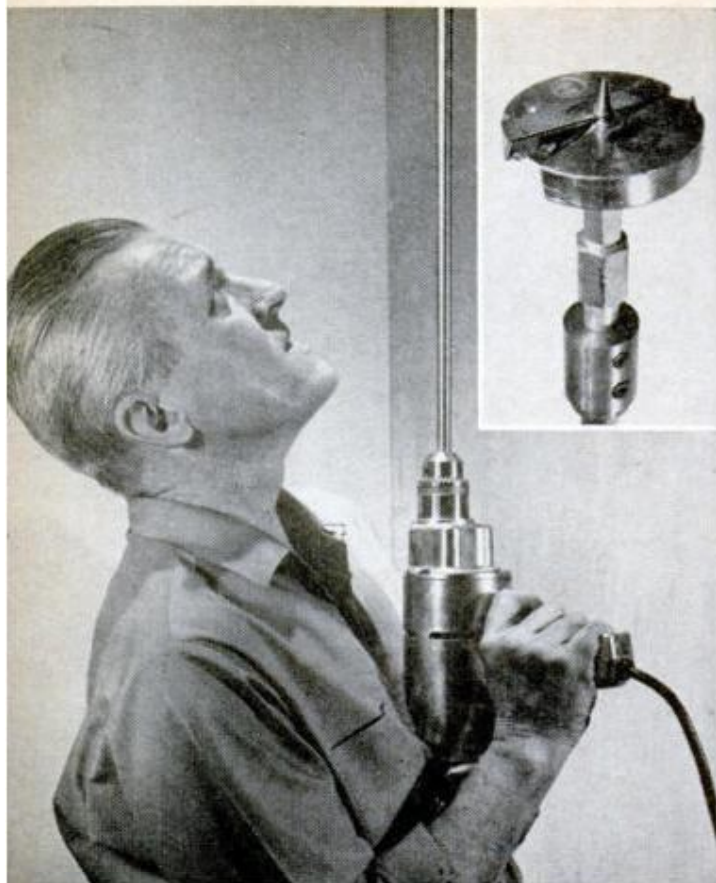
HOLE CUTTER (inset) at end of bit extension makes quick work of boring holes for tubing through floor and sole plate from below with a portable drill
