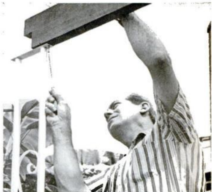
TRANSLUCENT ROOF , left, makes use of Filon fiberglass panels over an egg-crate framework. The front header is supported by decorative metal posts, above
