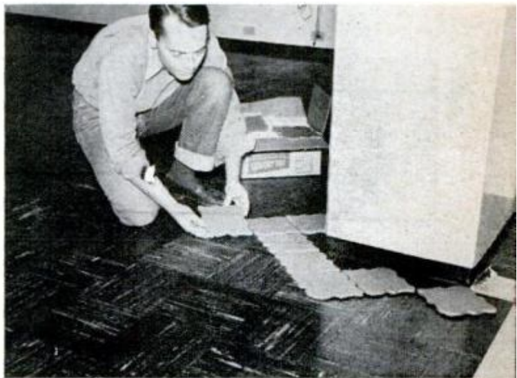
START LAYOUT at floor’s most critical spot, where tile pattern will be conspicuous. Here, whole tile are run around a corner toward threshold border. The floor boundary is masked with tape and foil
