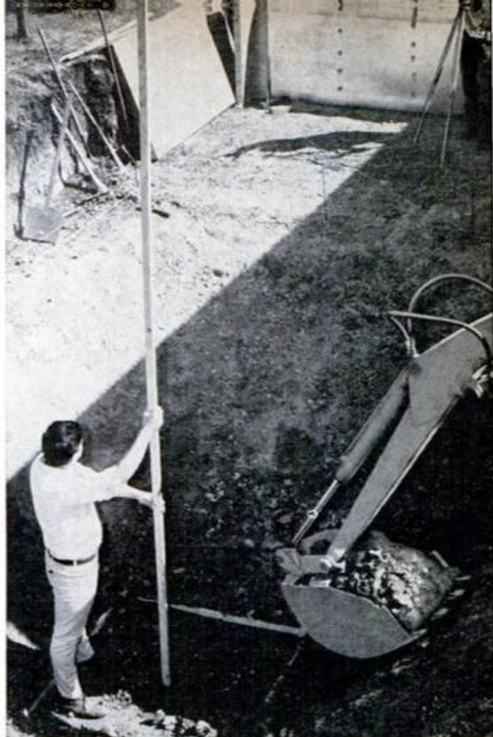
YOU HIRE this part of job. Backhoe digger does neatest job of shaping hopper hole at the deep end
