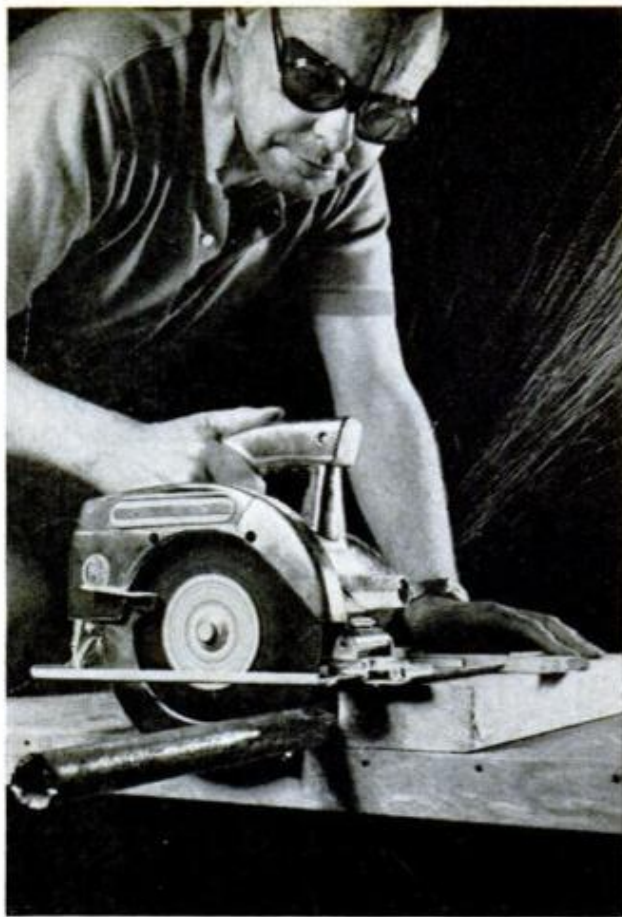
TO CUT PIPE , use abrasive cutoff wheel in a portable saw. Block the pipe between two 2x4s and tack a wood strip across the blocking to guide saw
