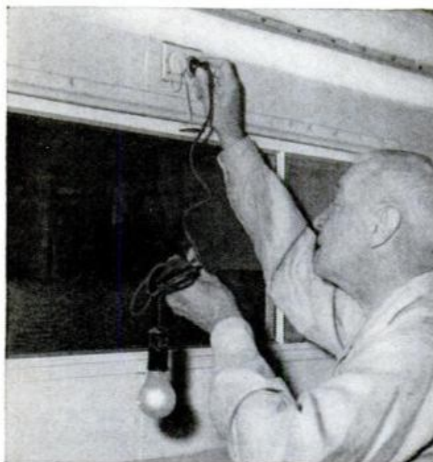
THERE'S ALWAYS A USE for an outside outlet. It's better to have it as high as you can easily reach. Low outlets could be fouled by water from wet roads
