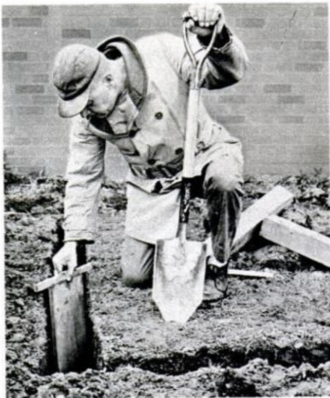
TRENCH FOR FOOTING is dug the width of a spade and to a depth below the frost line in your area. Uniform depth is assured with use of a T-shape gauge
