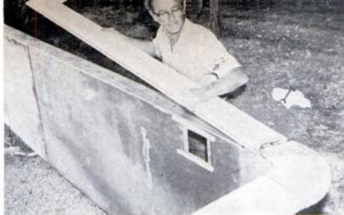
AFTER POOL WALLS are bolted together, white snap-lock coping is added around top of steel sections, fitting the corners first. Bolts in T-slots hold it
