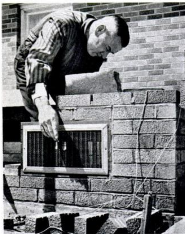
FOUNDATION VENTS are required to provide adequate circulation of air throughout greenhouse. Air enters through bottom vents, leaves through roof vents
