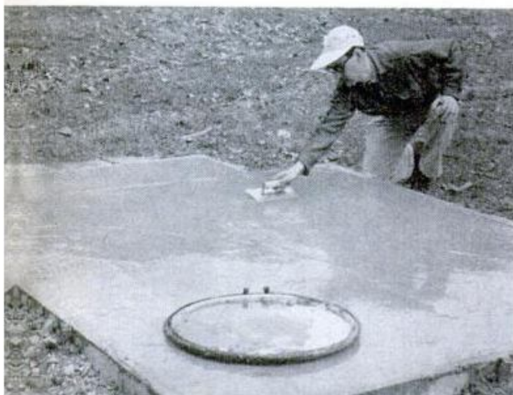
FINISHED SLAB , showing drum located a few inches away from edges at a back corner. Small depressed slab at opposite end serves as shallow step for entry
