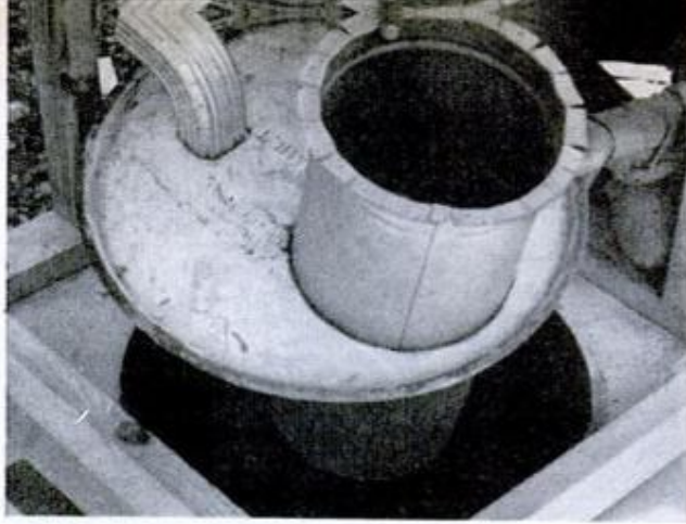
OPENINGS IN DRUM LID are cut for attachment of drain and downspout elbow and for slide fit with a length of 12-in.-dia. galvanized pipe hung from box
