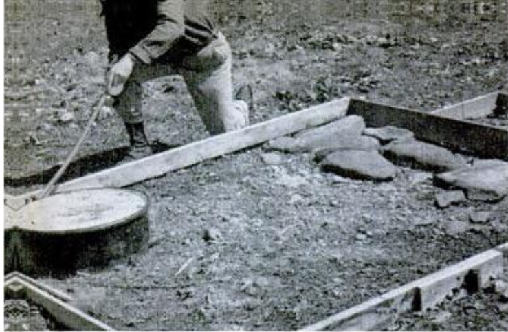
PREPARED OIL DRUM is sunk into the soil within 4 in. of the lip so that latter will come flush with top of concrete slab. Build 7x8-ft. frame for slab
