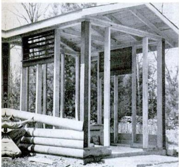
SCREENED LOUVERS are built into 2x4 framing at top of each sidewall. Siding in this installation matches that of cabin, but any handy material can be used
