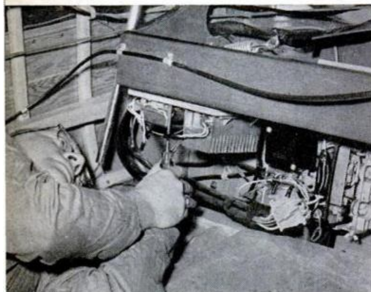
UNDER TRANSOM WELL is a good spot for mounting kit board, since it provides protection from spray
