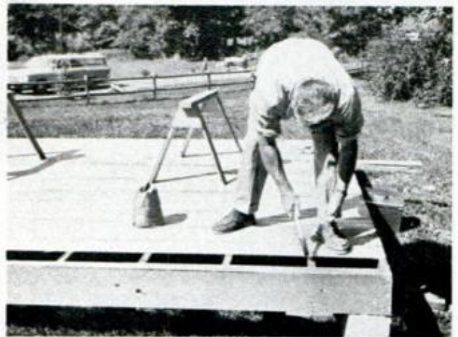
FLOORBOARDS ARE NAILED to joists while painted edges are wet. Standard 12-ft. boards are just right
