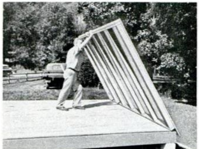
BACK WALL , plywood and all, is raised as complete section, spiked to floor, plumbed and then braced
