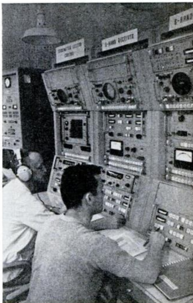
COMPLEX ELECTRONIC GEAR lines walls of "engine room" under antenna. Controls make possible sharp aiming of 9000-ton dish at targets far off in space
