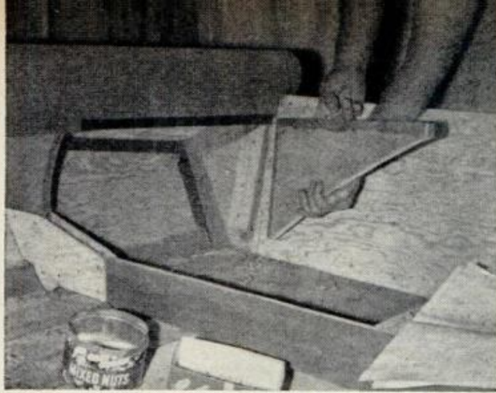
MOTOR-WELL KNEE fastens to carling, transom blocking and, for big motors, blocking on batten
