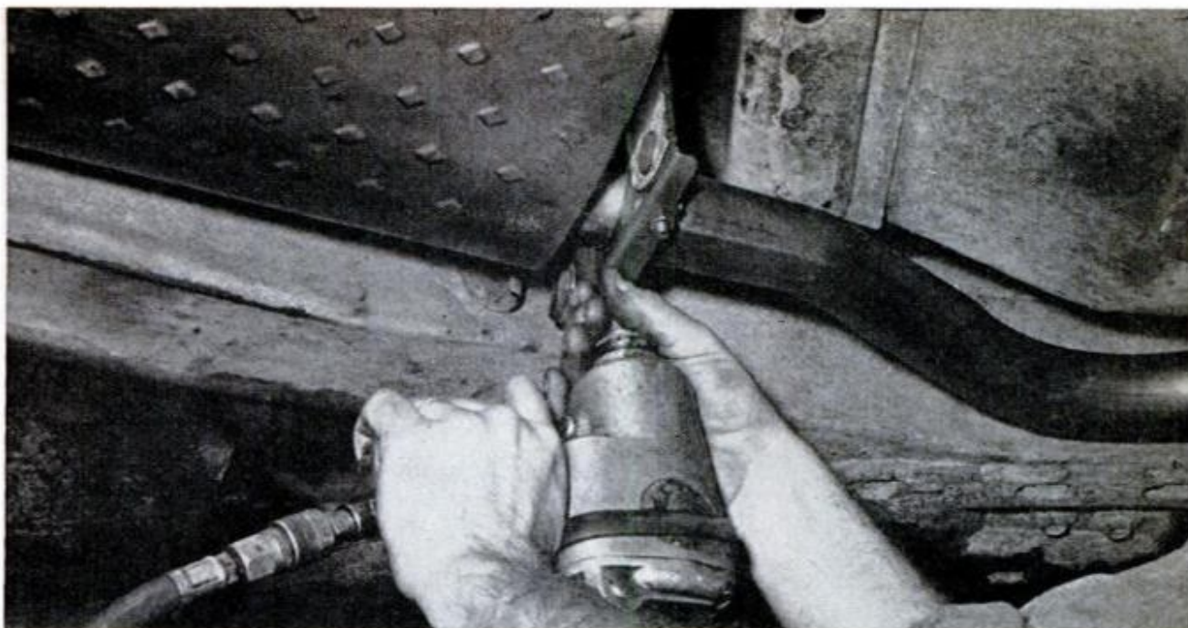
AT EVERY INSPECTION or whenever a part is replaced, all clamps and hangers should be tightened to prevent destructive banging of parts. This one, on a Chevrolet tailpipe, is a combination hanger and clamp
