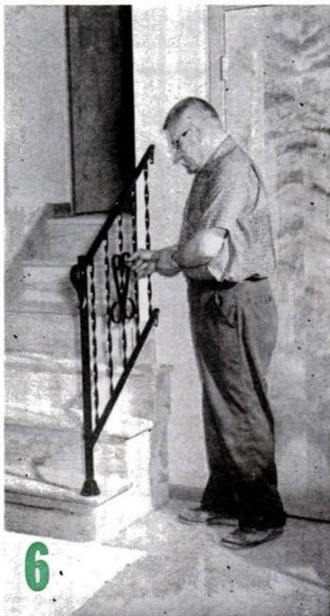
FINISHING TOUCHES are adding decorative scrolls to the balusters and curved endpiece to the newel
