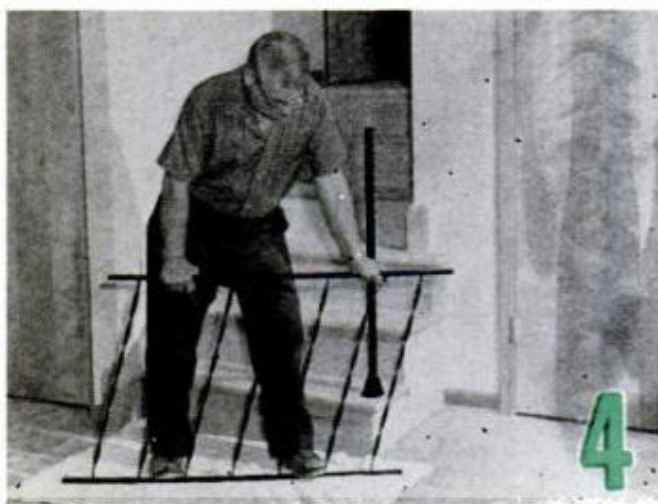
ANGLE THE RAILING so the balusters will be vertical when mounted. Place your feet on the bottom rail and press on the top rail, a little at a time, checking the angle against the pitch of the steps. Then cut the railing at both ends to keep equal spacing between the balusters and newel post. The cut must be angled the same as the slant of the railing
