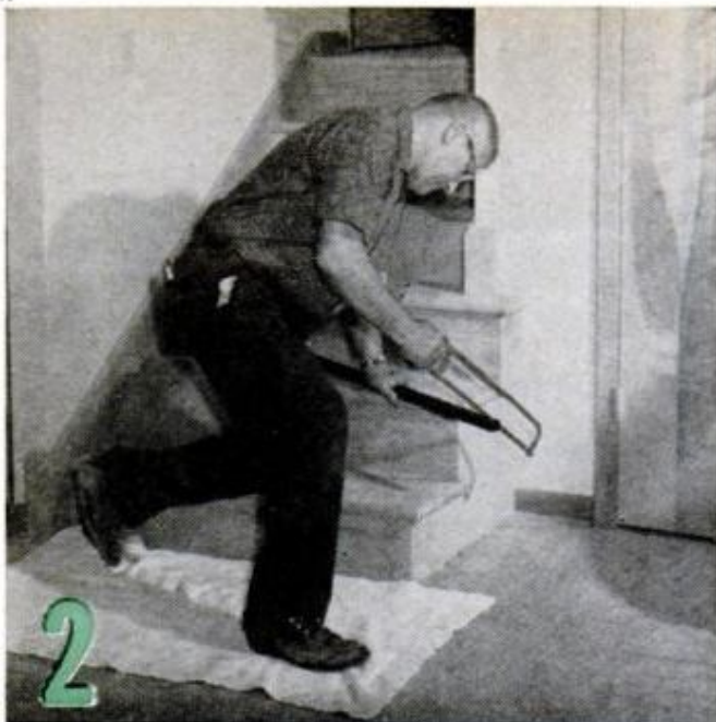
NEWEL POST IS CUT TO LENGTH at the bottom, depending on the railing height desired. Standard is 29 to 31 in. The cut need not be perfectly square
