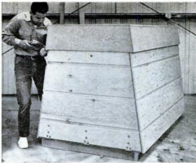
ROOF FITS OVER tapered sides of hut like cover of a box and serves to hold hinged front shut without catch
