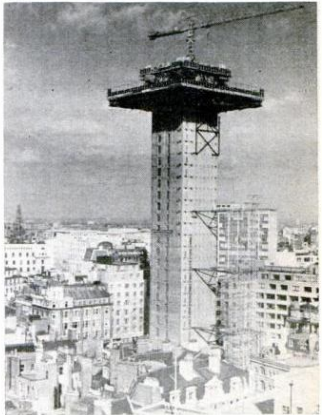
Built from the top down , a London office building rises—or sets—in the heart of the business district. The elevator and stair shafts were built first, then an overhanging platform was erected and the framework and floors were constructed from the top floor down. When the building is completed the platform will be removed.
