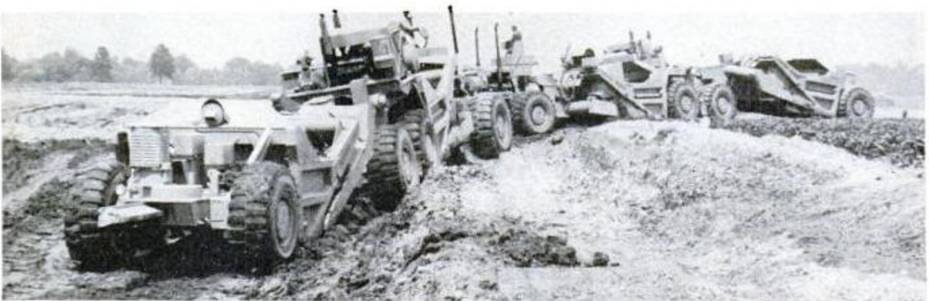
FIVE UNITS of electric digger, operated by one man (arrow) can pick up 150 tons of dirt in minutes
