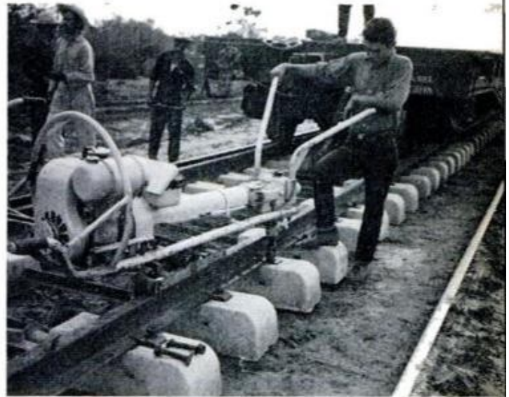
FRENCH TIES were used over most of route. Steel plates are placed on impregnated ties and covered by cushion of rubber before long rails are screwed on
