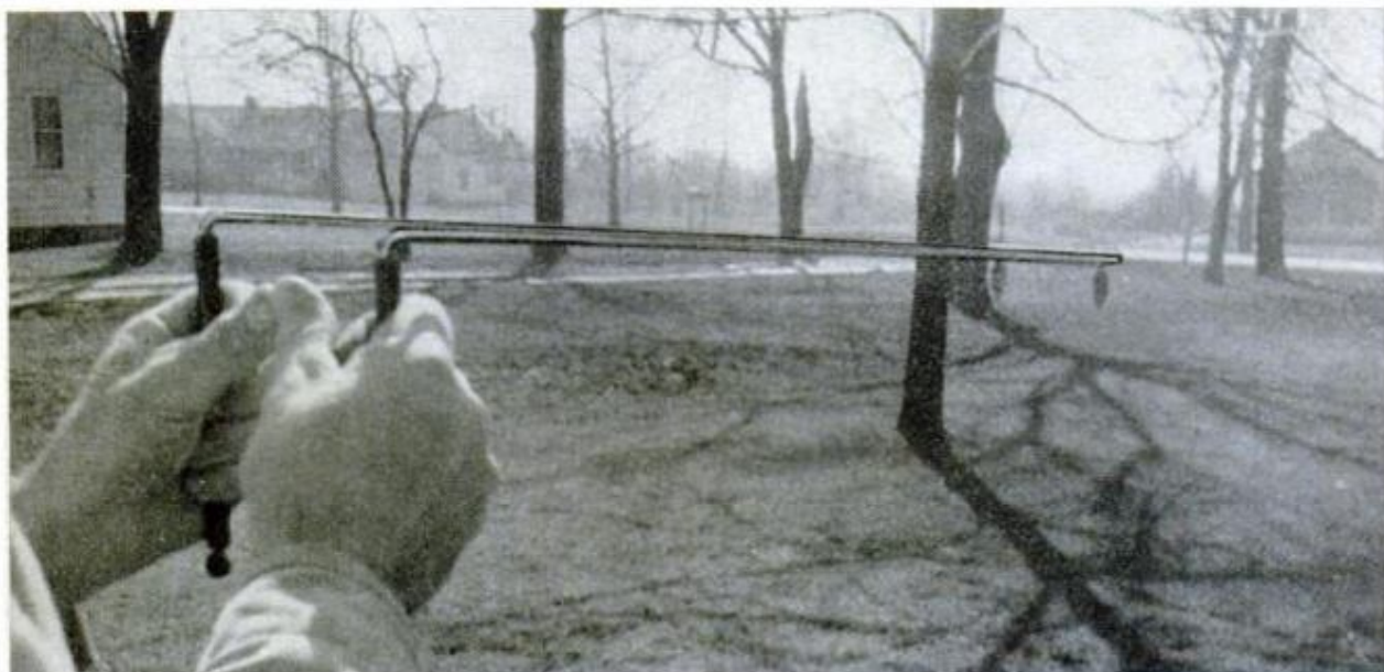
UNDERGROUND PIPES AND CULVERTS are sought out by rods in hands of Duke Diebold, water superintendent of Sheffield Lake, Ohio. "They've often saved us from excavating large areas," says Diebold
