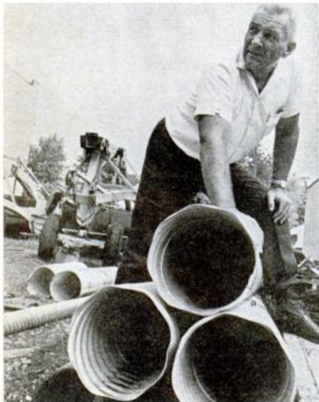
ALUMINUM PIPES that Krekel Karch straddles are installed in base of dike to provide drain for water that might otherwise remain on land too long
