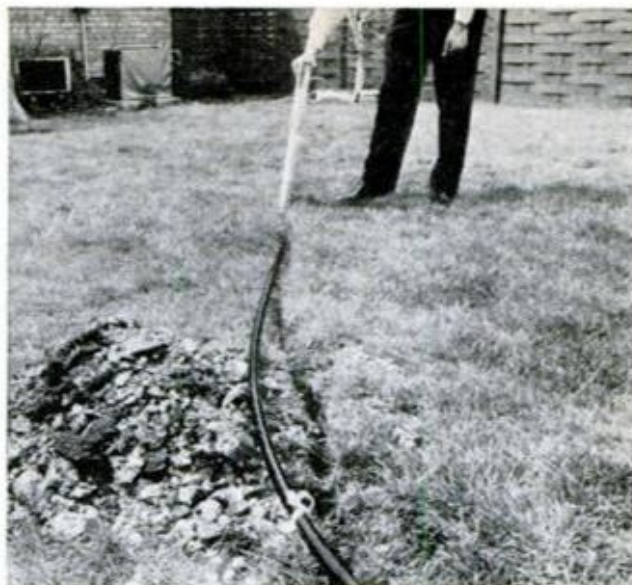
TRENCH CUT FOR HOSE leads to stake, where sprinkler in Sears Sprinkler-Matic system will be installed. Single head can water area 80 feet in diameter
