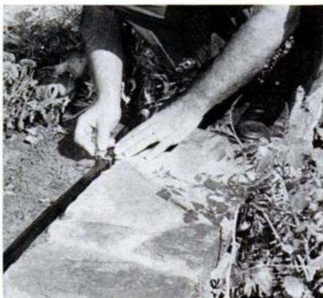
SQUARE-SHAPED HOSE is secret of new sprinkler system designed for foundation and border areas. Anchor spikes hold hose. It's sold by Sears, Roebuck
