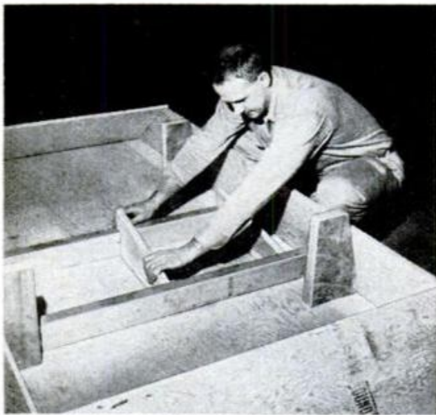
TEMPORARY BRACING is provided by angle brackets. Tacking end panels in place serves the same purpose
