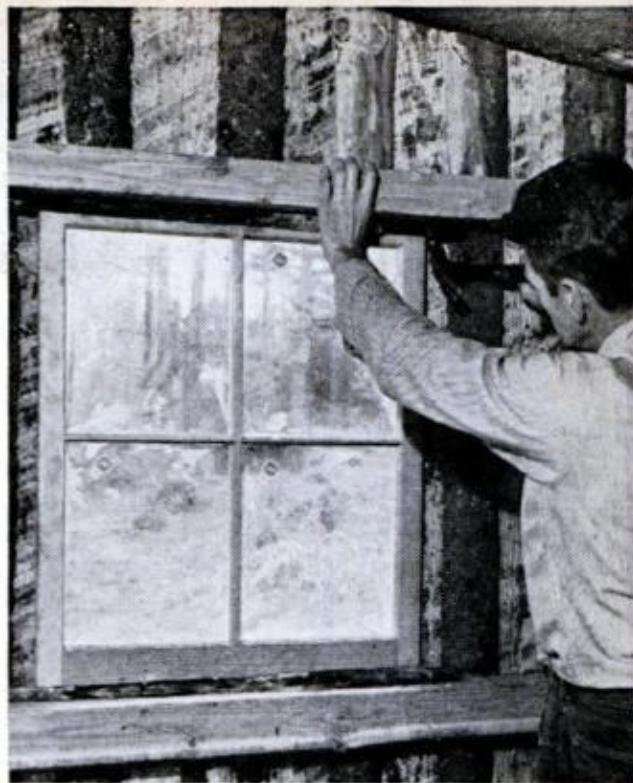
24. FASTEN WINDOW SASH in place with nails driven into horizontal framing members, then caulked to make it weathertight. Note interior battens are already applied to cover gaps
