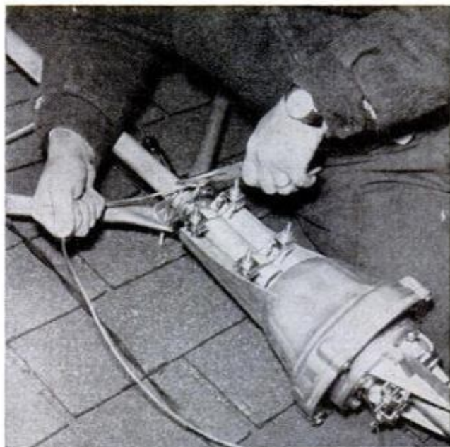
GUY WIRES go to a guy collar if rotator does not have provision for attaching guy wires, or if additional support is needed. We did both to show how
