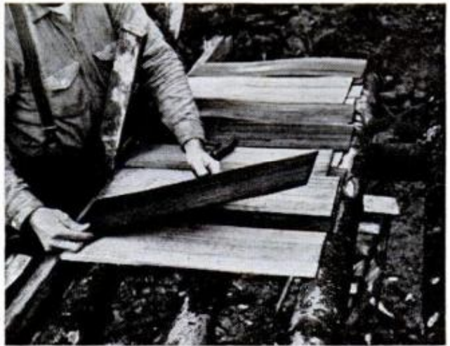
SHAKES are laid across the purlins to form roof. Shakes were made for this roof by cutting cedar log into 25-inch bolts; wood mallet and shake froe then were used to split bolts into shakes
