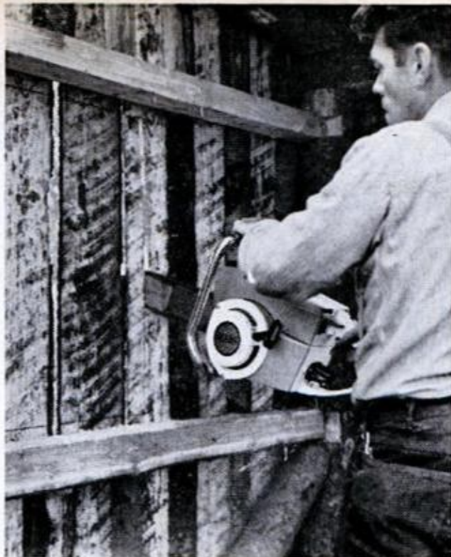
23. CUT WINDOW APERTURE after the siding is on. Window used in pilot model is a 28 by 30-inch nonmovable frame, though you can use any size by first adjusting framing height
