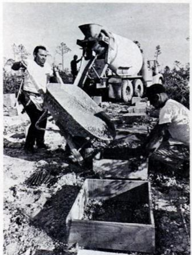
WITH FRAMES SPACED , in place, concrete for 24 pilings is poured. Pilings support foundation beams, which go in place when concrete dries
