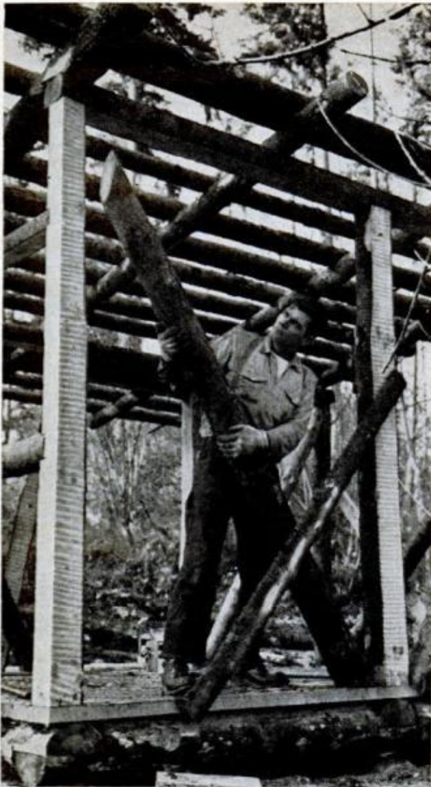
PERMANENT CROSS BRACING goes into place between the upright posts, as shown here on rear wall. Ends of the bracing logs should be cut at angle to fit upright and floor
