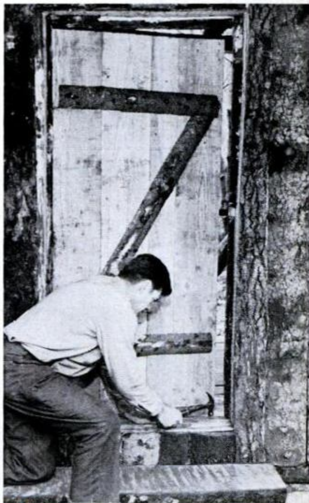
26. DOOR PLANKS are ripped from 10-in. log, and slabs form the cross braces. Fence is made of three 10-inch posts sunk in ground four feet apart. Braces, ripped from six-inch logs, are 3x6 in.
