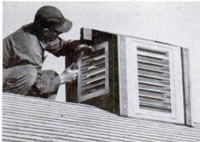
NAILING LOUVERS IN PLACE must be done before adding roof since overhang would interfere. Either aluminum nails or screws can be used to fasten them
