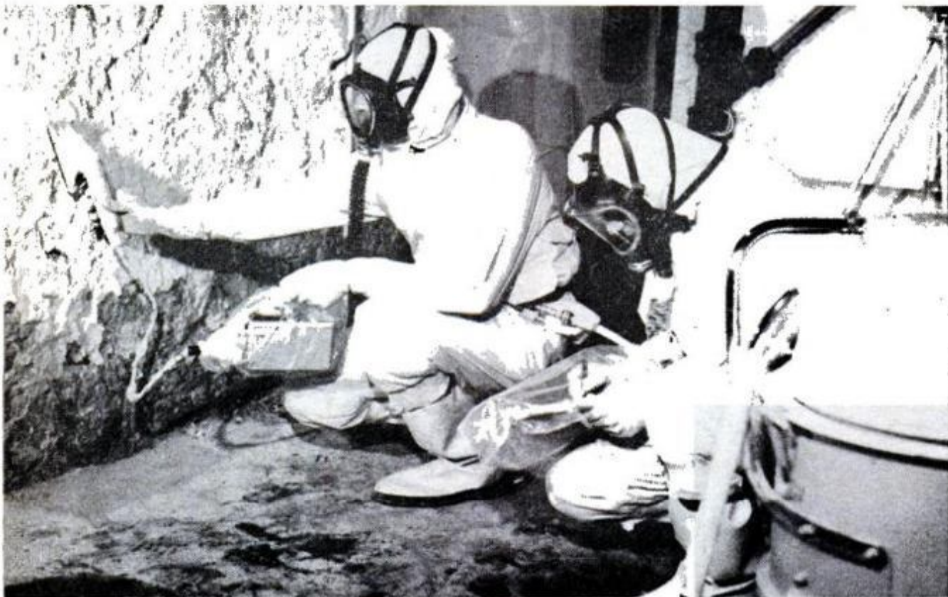
CONTAMINATED WITH RADIUM , basement of home in Lansdowne, Pa., is surveyed by crew in protective suits
