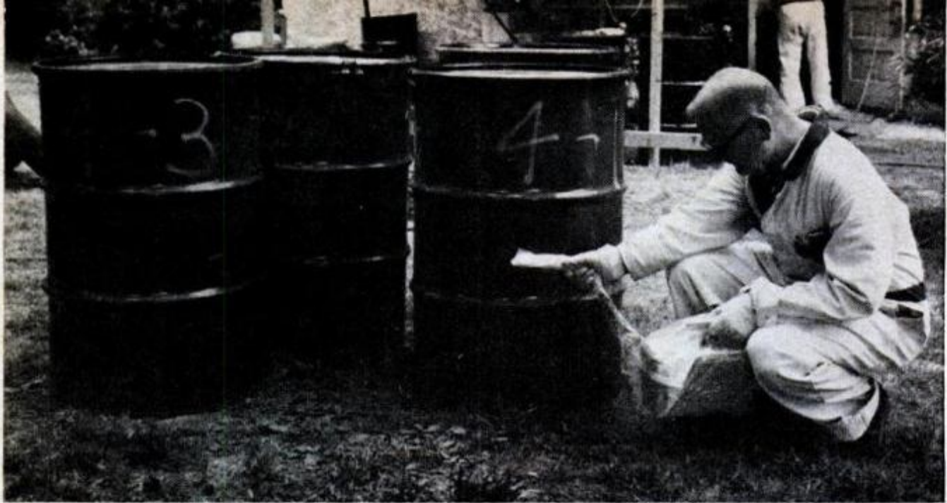
CONTAMINATED MATERIAL from Lansdowne house was removed in drums and shipped to special burial site. Total of 180 55-gallon drums containing about 30 milligrams of radium was removed during 3½-month project
