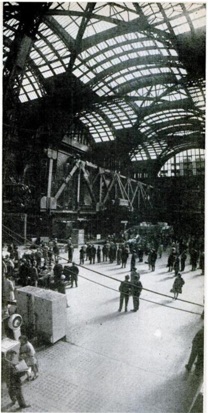
GIANT TRUSS THAT WILL SUPPORT section of new center runs right through Penn Station's big concourse. It's anchored on steel "legs"
