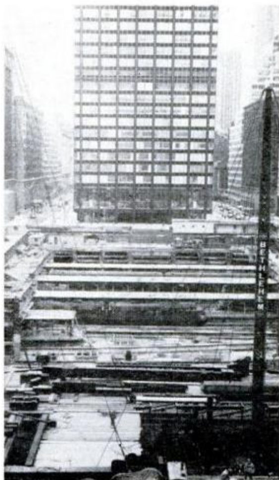
A SIMILAR CONSTRUCTION PROBLEM was involved in putting up a big office building on New York's Park Ave. Trains continued to roll while the steel foundation was put in place
