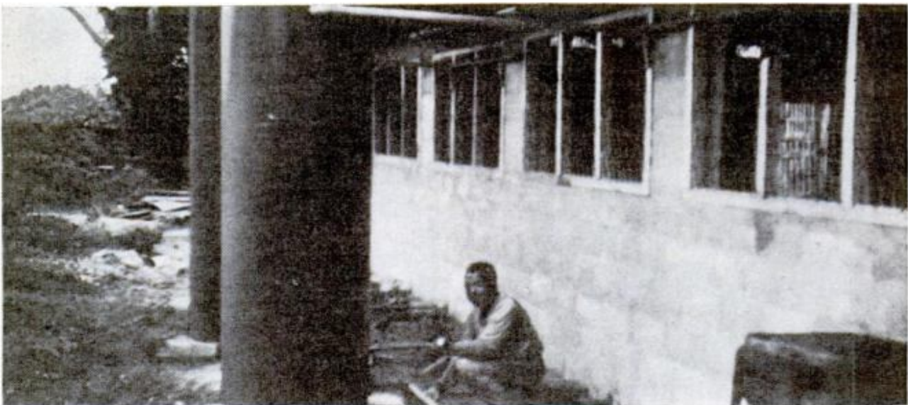
TYPICAL SCROUNGING operation used discarded cable spools as cooling tanks for diesel engines. Welded together, they formed 12-foot tanks. Steam pipe from engines entered bottom of tanks and, rising through water-filled tanks, the steam cooled as it rose, returning to engines from top of homemade, improvised tanks
