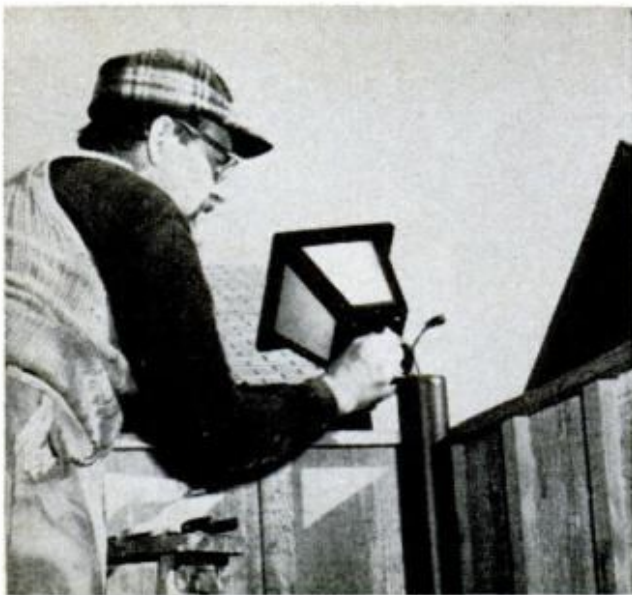
WIRING POST LAMPS is simple matter of twisting and taping leads from fixture and wires you previously ran up both posts; soldering is optional
