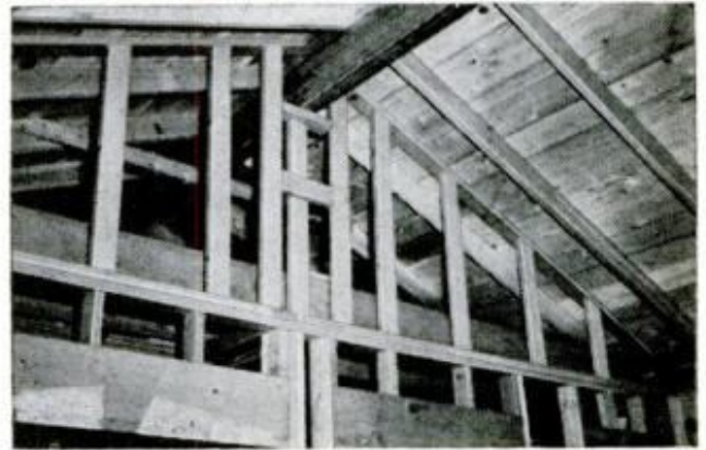
GABLE FRAMING of patio wall has studs installed sideways for easier toenailing to under-roof cleat. Note beam support ties into framing for 12x12 vent
