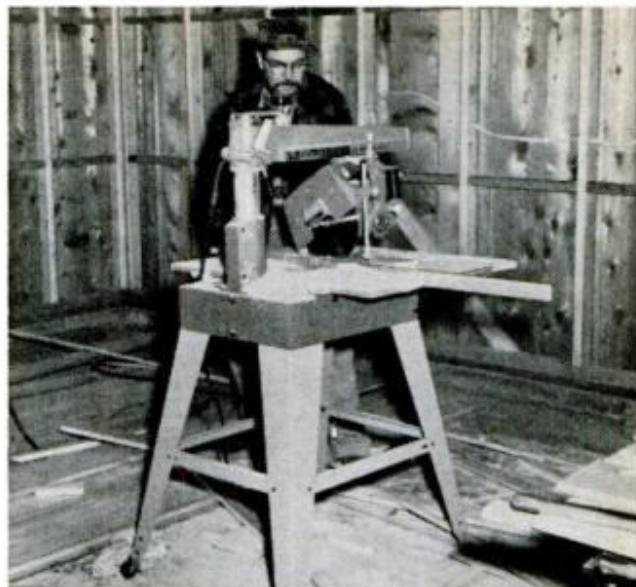
FINISH WORK goes on in all weather if you move your radial-arm saw inside after your wiring's in. Mine will stay here as the nucleus of my new shop
