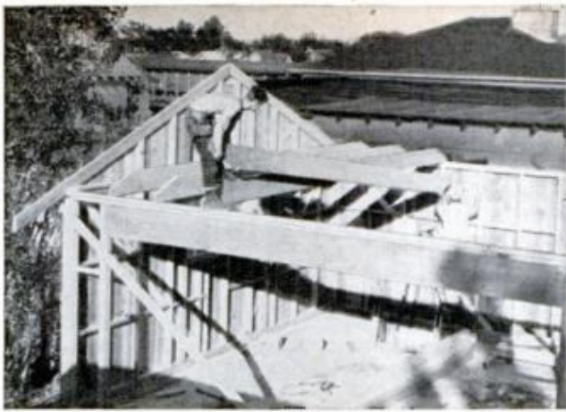
POSITIONING JOISTS is two-man job. They rest on—and are nailed to—top plates of eave walls and are spaced 24 in. o.c. End bevels match roof pitch
