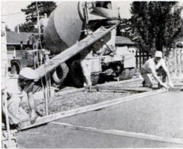
BECAUSE DRAINPIPE and waterline stick up, rod off to this point along patio, then fill rest of form
