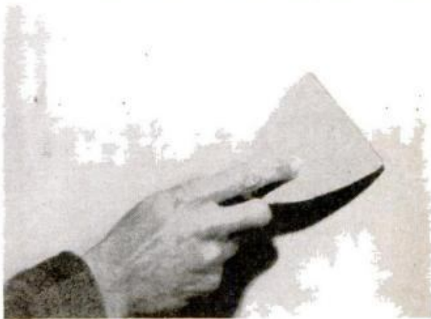
TO CONCEAL PATCH, let initial coats of cement dry, then follow with two more coats, as on joints
