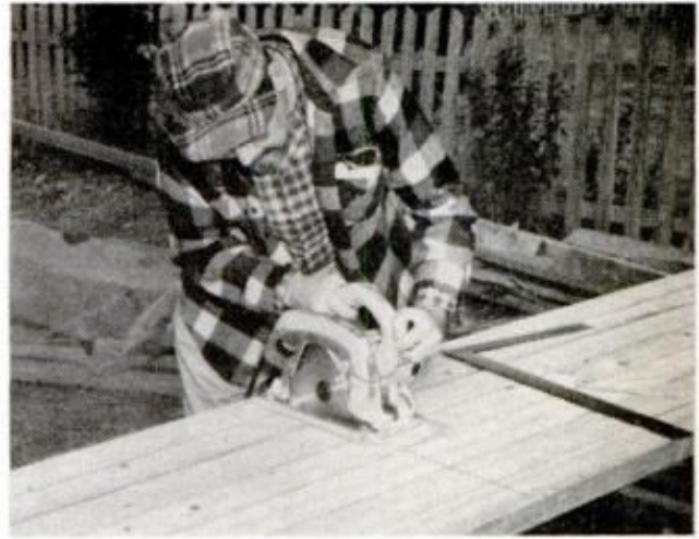
PORTABLE CIRCLE SAW makes fast work of gang-cutting studs from 16-ft. 2x4s laid edge to edge and scribed across with a carpenter's square, above
