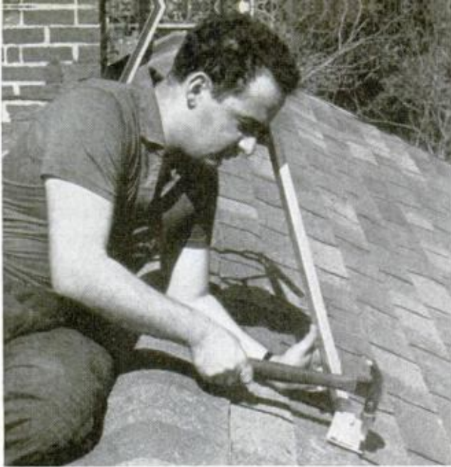
START MOUNTING BOLTS with a hammer. Be sure they are going into the rafters for a firm solid grip. Cover with silicone rubber or tar to prevent leaks
