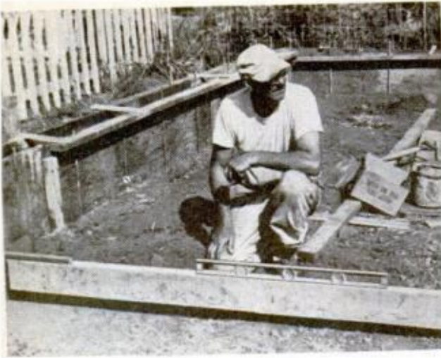
LEVEL FOUNDATION FORM at door gap by hanging plank between bulkheads, adjusting them till it's level
