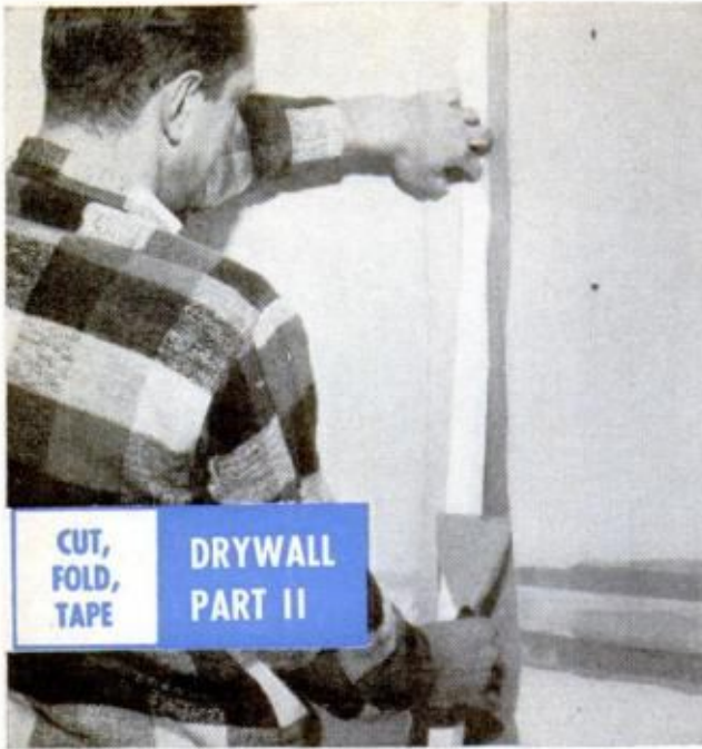
TO TAPE INSIDE CORNER , fold tape down its center, then press it into corner with knife or corner tool
