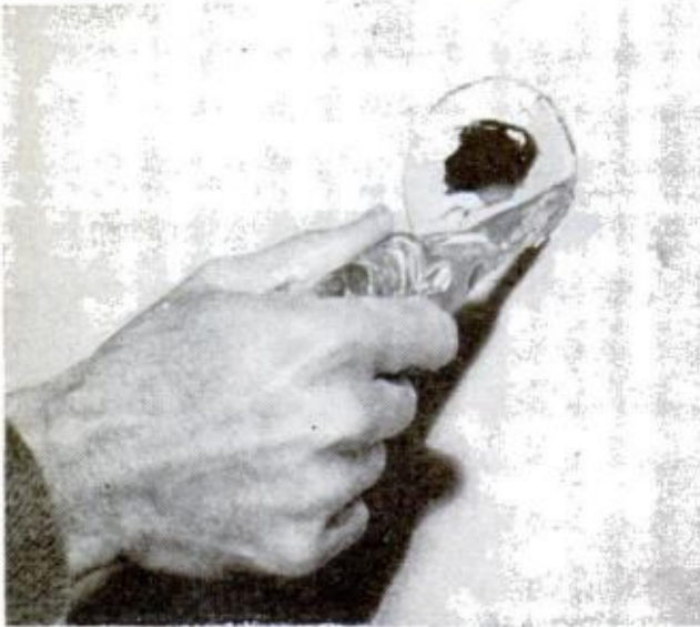
FIRST STEP IN PATCHING a small hole is to draw 3-in. or larger circle around it, then cut out circle
