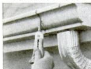
Fix gutters, windows
