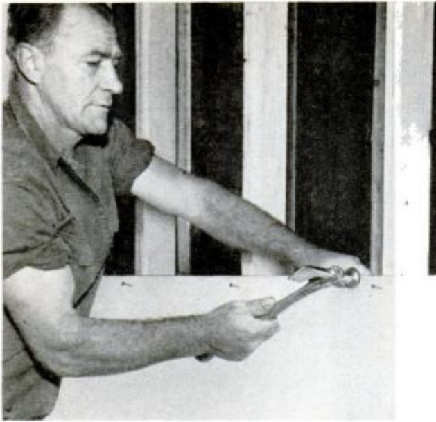
BEFORE LIFTING WALL PANEL into place, lean it against studs, right under its final location. Use stud centers to position nails along top edge of panel
