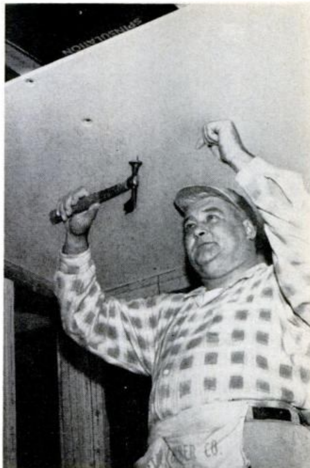
IN NAILING CEILING PANELS, a backhand hammer stroke gives a clear view of nail heads. This permits accurate aiming of strokes, lets you line up nails by eye. Workman is supporting panel with his head
