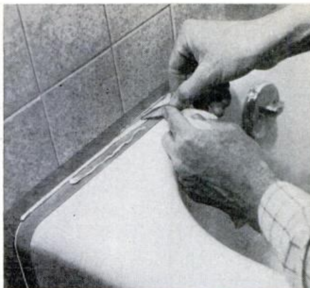
AFTER TRIMMING with stick as shown in sketch far left, pull up masking tape. Excess comes up with it to leave smooth, permanent tub-tile joint
