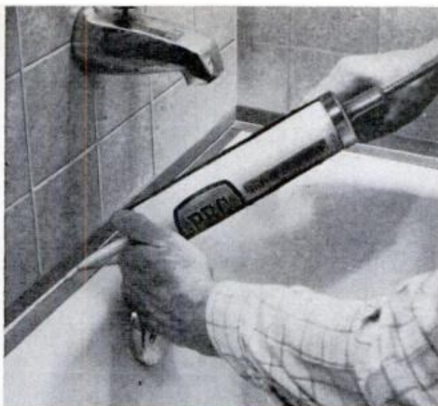
SIMPLIFY CLEANUP by applying masking tape to both tub and tile. Trim plastic nozzle of disposable tube at angle and squeeze sealant well into gap
