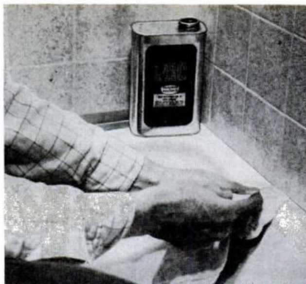
AFTER REMOVING cracked grout between tub and tile, wipe tub clean with solvent-soaked cloth wrapped around putty knife and inserted under edge of tile
