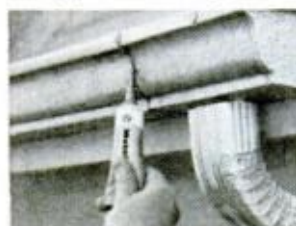
Fix gutters, windows
