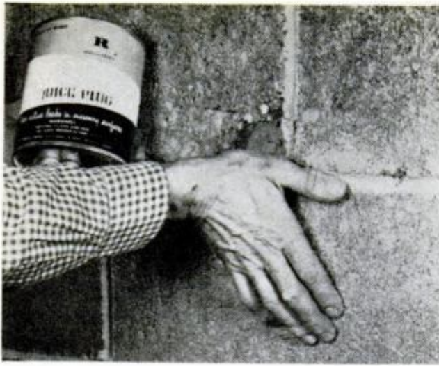
ANOTHER FILLER for cracks or big chips is a putty-like compound. It's tricky to use because it dries in 3 to 5 minutes after you mix it with water. Roll it into a ball, slap it into crack and trowel smooth
