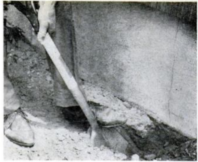
EXTERIOR CRACK often extends far below grade. You must uncover and patch the full length; it does no good to patch the upper visible section if water will continue to leak through the underground part
