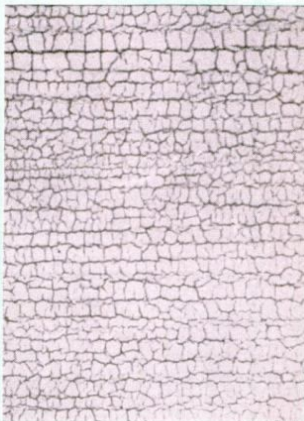
HERE'S WHAT CHECKERING (also called alligatoring in advanced stage) looks like. Caused by cheap paint or insufficient drying time between coats
