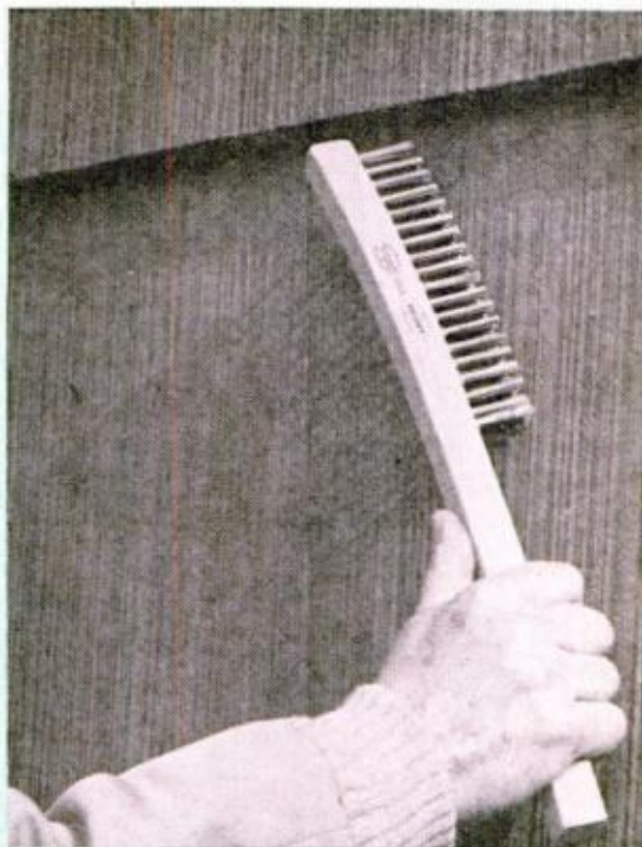
DON'T SLIGHT on the preparation of the surface in your eagerness to get started. Wire brush areas where the paint has peeled or blistered
