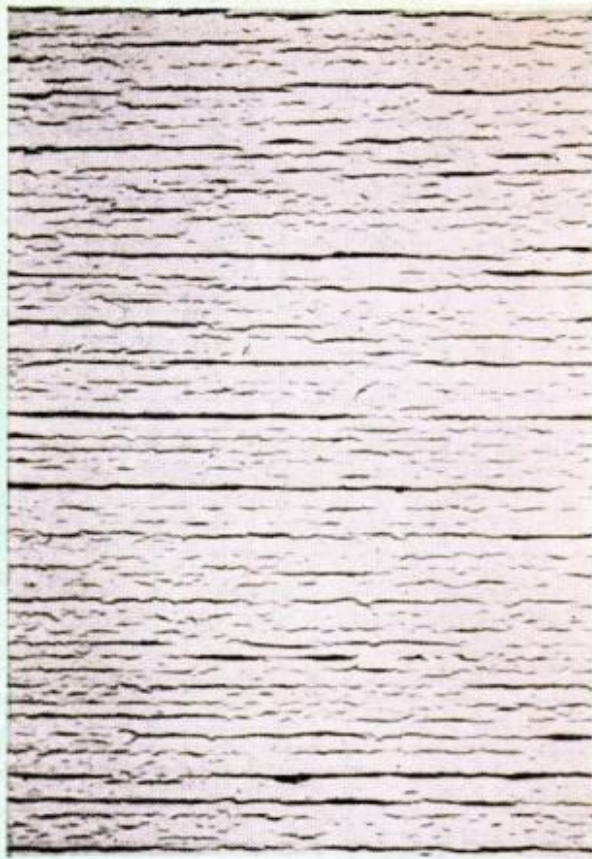
ADVANCE STAGE OF CRACKING where deep cracks in paint extend down to the bare wood
