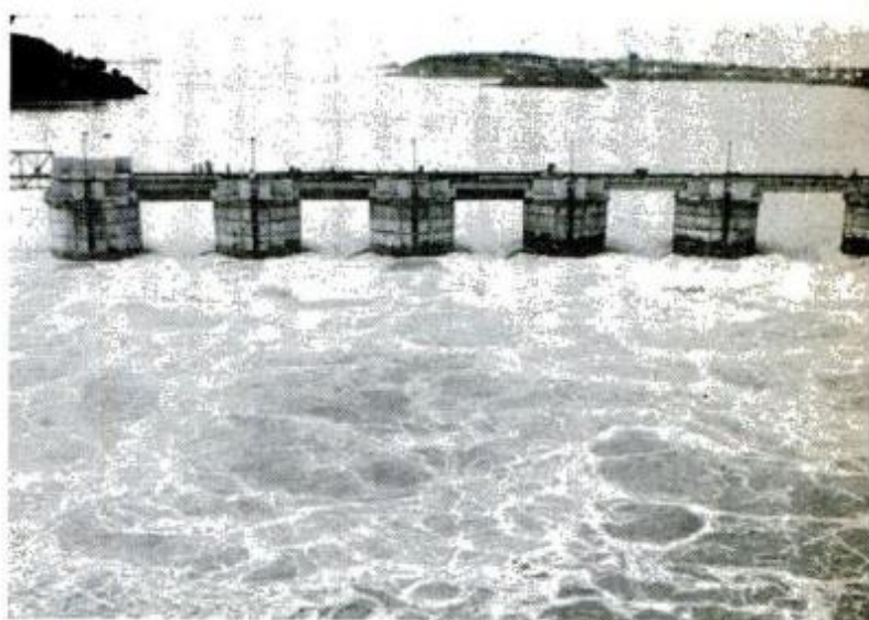
UNCONVENTIONAL CYLINDERS of prefabricated reinforced concrete were set up like picket fence, then gaps between them were filled in to make cofferdam
