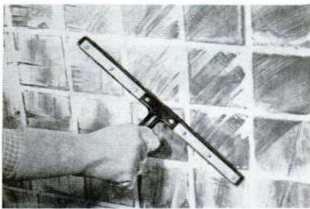
AFTER ALL JOINTS have been filled with grout, wipe off all excess grout with a common window squeegee
