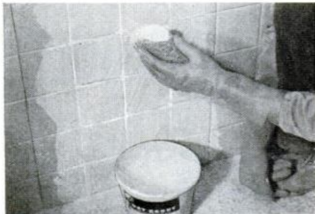
GROUTING is the final step. Mix the powdered grout with water to form a paste and sponge it over tile
