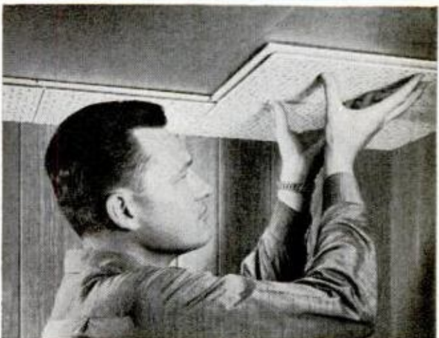
STARTING FROM CORNER , each tile is placed \frac{1}{2} in. from final position and pressed within \frac{1}{8} in. of ceiling. Then tile is moved until its tongues engage grooves of already-placed adjacent tiles
