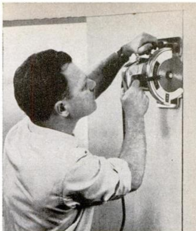
ENLARGING EXISTING OPENINGS —whether for a pocket door or a bigger window—is quickly done with a cut-off wheel in electric handsaw. Slice through both sides before you chop away plaster and lath
