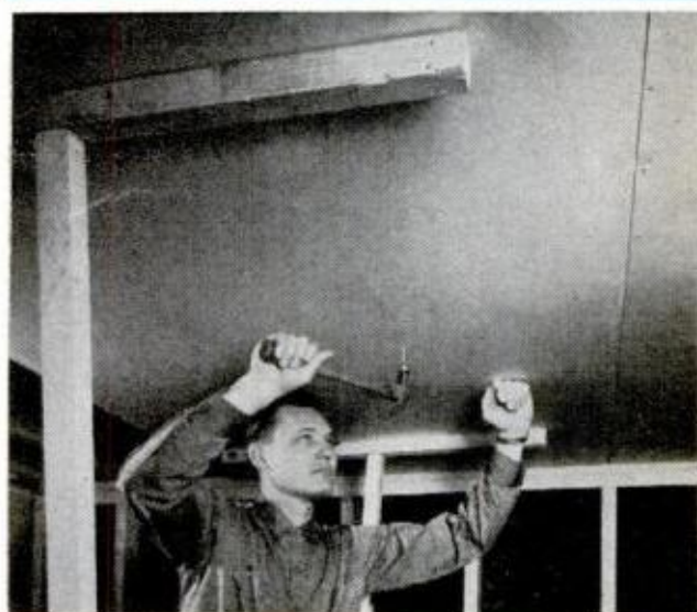
BIG WALLBOARD PANELS cover joists fast, can be handled by one man with the aid of T-braces made by nailing 2x2s together. Long edges should be centered on stud, nailed every 6 inches
