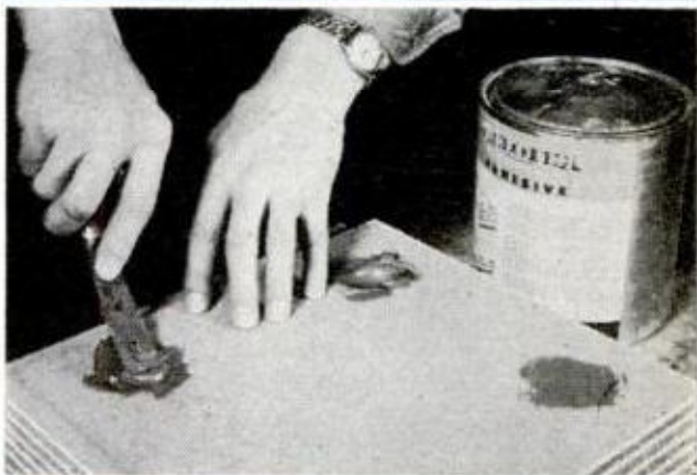
HEAVY-BODY ADHESIVE is placed in walnut-sized dabs on 2\frac{1}{2} -in.-dia. spots primed at corners of tile (right foreground). Special cement eliminates stapling required with light, slow-bond types
