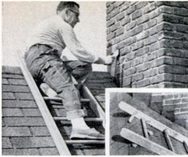
FOR ROOF PERCH , lay ladder flat, hooking brackets over ridge (inset). This simplifies climbing up and down, gives you choice of levels from which to work
