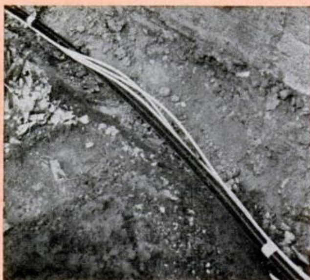
CONTROL LINES for the hydraulic valves should be run in the same trench as the pipe where practical
