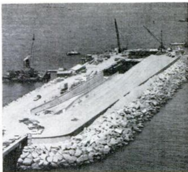
ISLANDS TO CONNECT TUNNELS were built in 30 to 40 feet of water by creating a 22-acre pile of sand and rock reinforced with concrete dikes. Center of each island is the entrance to the mile-long tunnel
