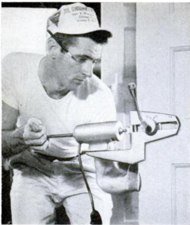
COMBINATION boring jig and power tool makes possible rapid installation of cylindrical locks in house doors by the builders of development houses
