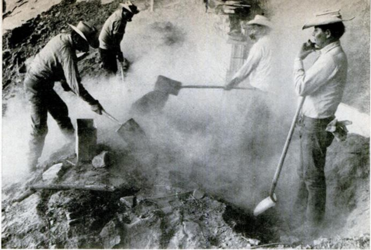
ADDITIONAL HAZARD was fumes from dust and fetid remains of centuries-old garbage uncovered by excavations. Workers wore respirators to avoid infection while digging trench to lay new foundations
