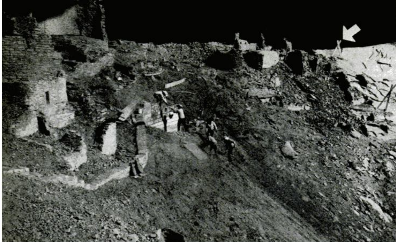
WORKING CONDITIONS were hazardous because cave sits on top of slope high above canyon floor. Mortar was hauled up from bottom by cables strung over scissor braces (arrow). Navajos are repairing retaining wall
