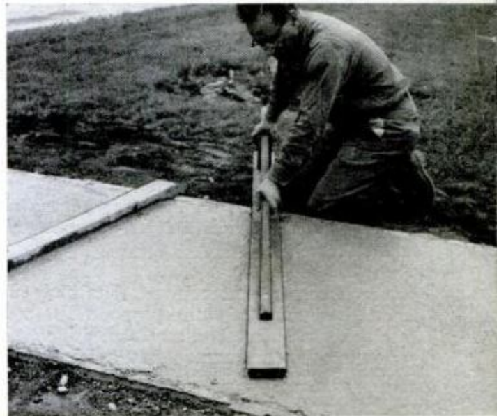
PRESS STONES into concrete until they are covered by thin layer of cement paste. Then apply retarder
