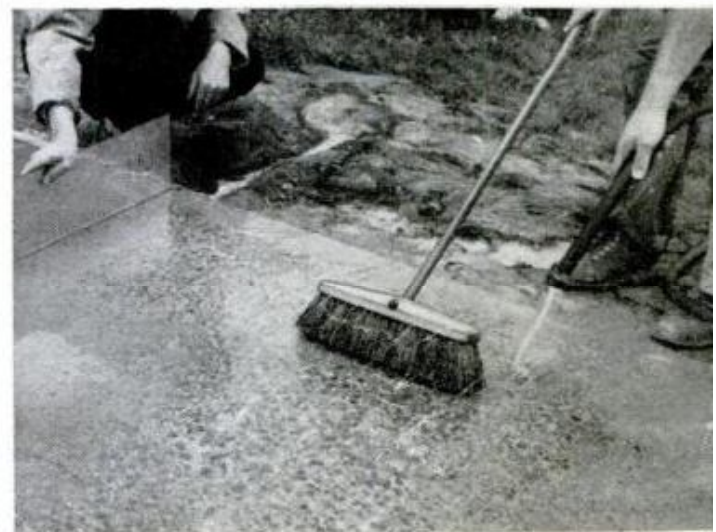
BROOM THE SURFACE lightly and wash away cement paste with light stream from hose exposing the stones
