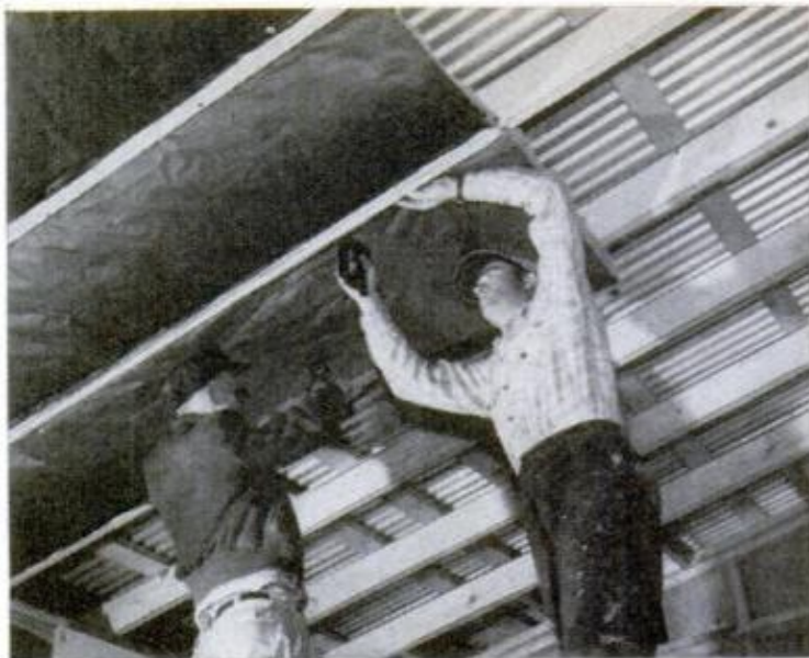
BAT INSULATION in 8-ft. lengths is being installed between roof rafters. The flanges are stapled to the sides of rafters
