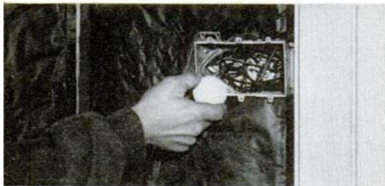
TO SPOT LOCATION of outlet box on back of paneling, chalk edges of box and press panel against it
