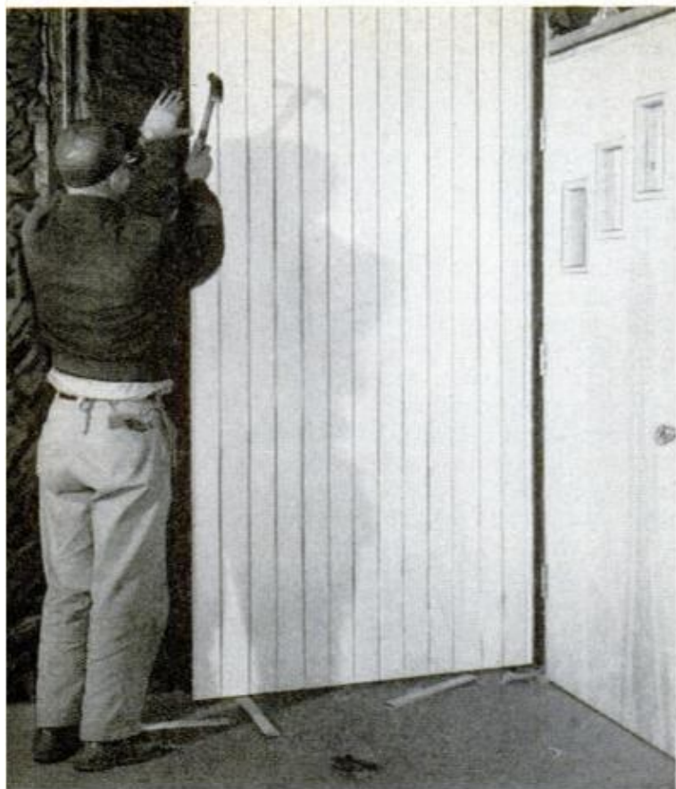
VERTICAL-GROOVED HARDBOARD paneling was used in pilot home. Here first panel is started in corner
