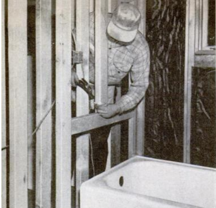
AT FAUCET END of tub, left, stud is shortened and a header installed to permit plumbing connections to tub
