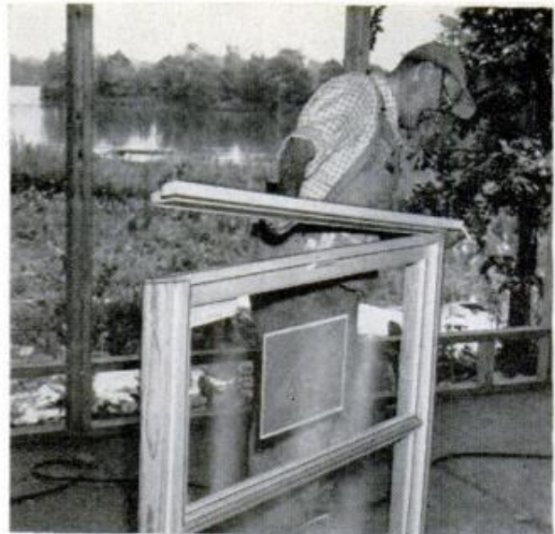
KNOCKDOWN WINDOW UNITS are assembled on the job prior to installing in openings in prefabricated walls
