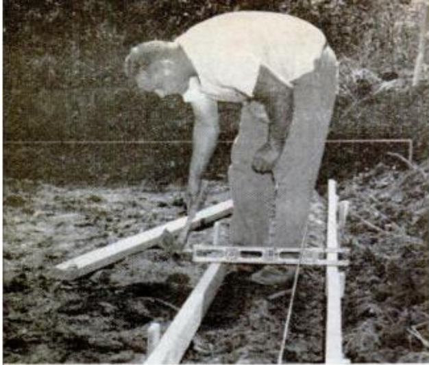
FOOTING FORMS are 2 x 4s, set on grade, then dug out for an 8-in. poured footing
