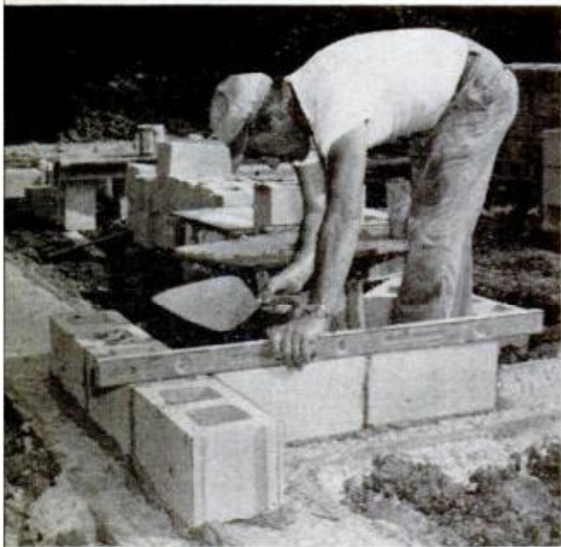
STUB TIE-INS are laid at corners of basic foundation when future addition is planned
