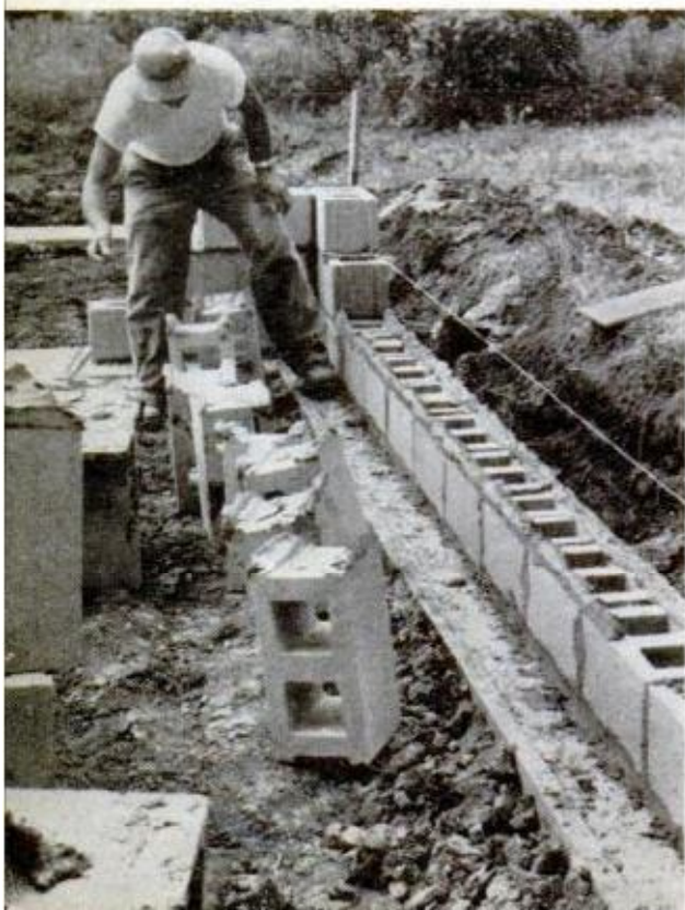
FOUNDATION GOES FASTER when several concrete blocks are buttered at same time
