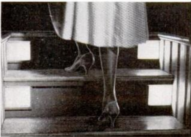
SOFT, GLARELESS LIGHT from electroluminescent panels keeps stairways easily visible and safe all night. The Rayescent panels are available for $8.40 each from Solar Sonic Devices, Inc., Hicksville, N.Y.
