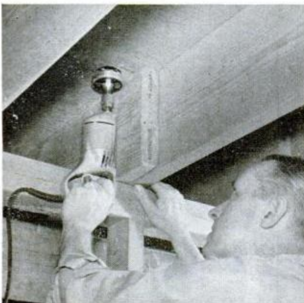
8. HOLE SAW in portable electric drill is used to bore holes up through floor for passage of suction ducts
