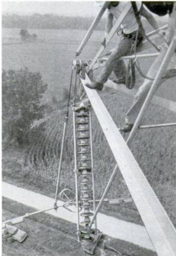
FIRST FEAR lineman must overcome is not fear of hot wires, but of heights. He spends year of on-the-ground training just learning hot-wire techniques
