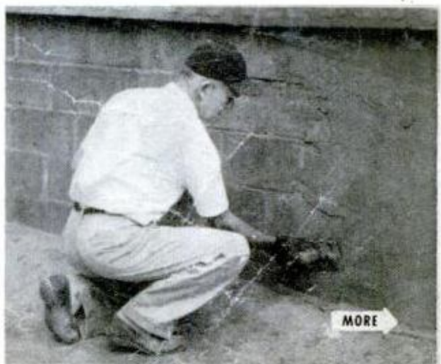
WALL IS CEMENT-PLASTERED with specially prepared waterproof mix and is finished with masonry paint
