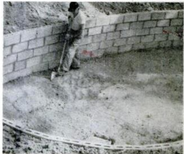
DIVING AREA is dug out after pool walls are laid up. Earth excavated is later used as fill outside walls
