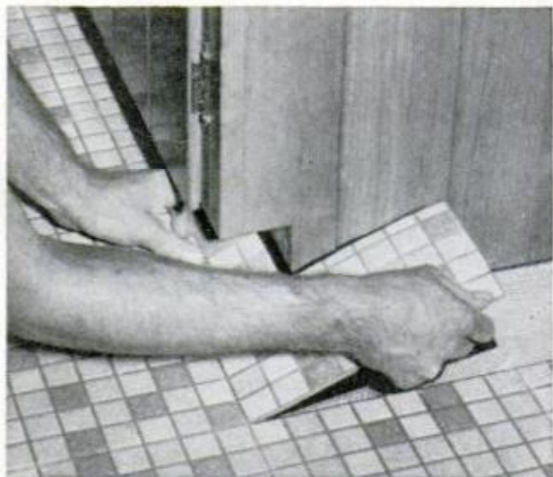
STEP 7. Nipped edges of border tile that will not be covered by base shoe, or quarter round, must be ground smooth before pressing tile in position
