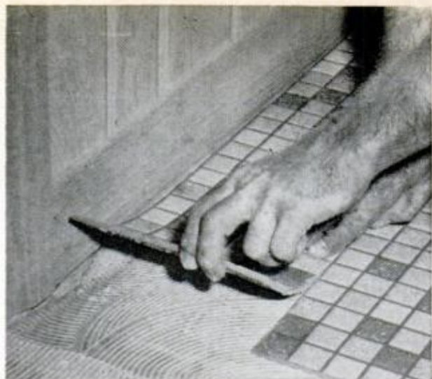
STEP 5. Job of cutting border tile is easy when it can be cut through rubber grout line. Insert tile as close as possible to final position and press down
