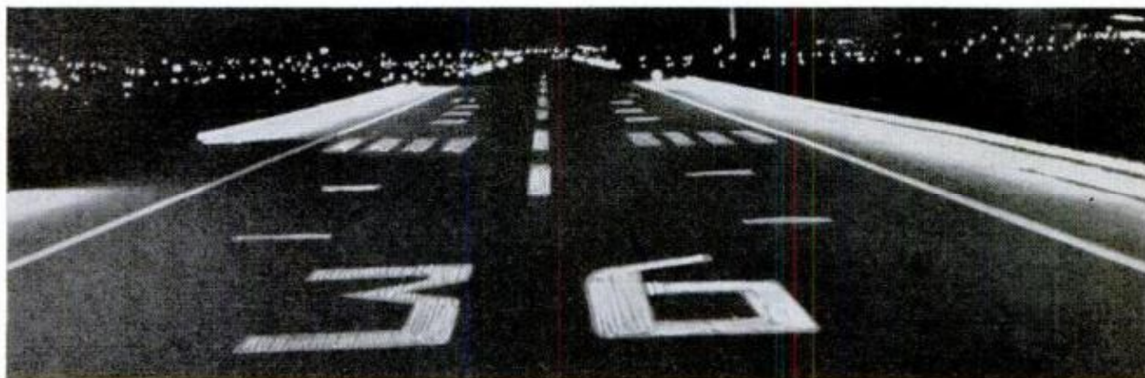
Modern lighting system, installed at Washington National, gives incoming pilot well-illuminated target
