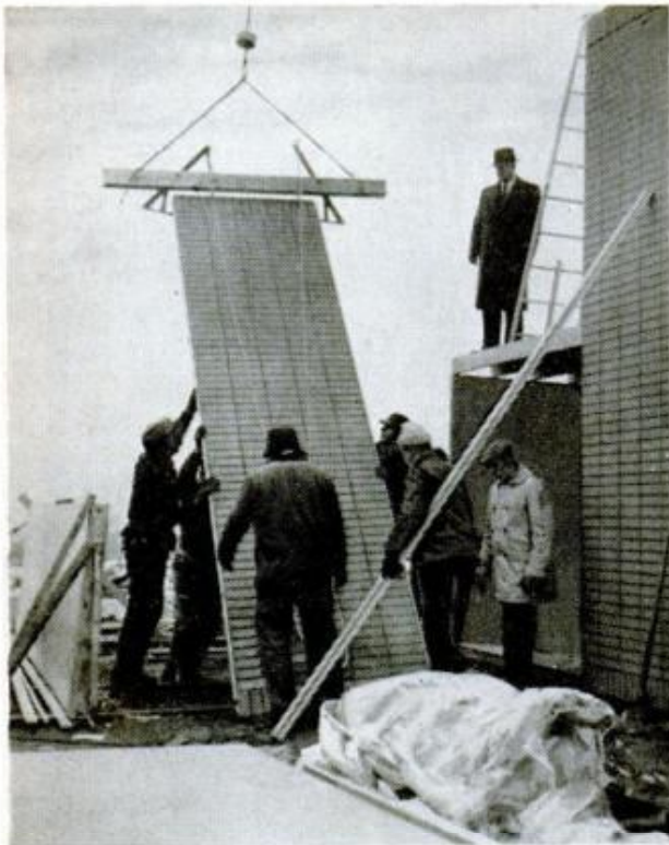
Foam-core, load-bearing wall has face of lightweight powdered brick, reconstituted to resemble brick veneer
