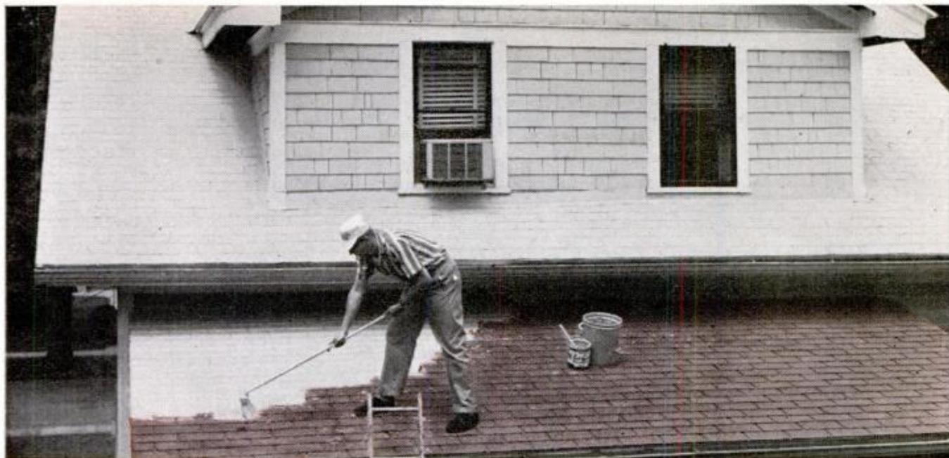
Arthur Behn brushes on a new pebble white roof with Foil-Gard Aluminum Paint, a product of the R. F. Johnston Paint Co., Cincinnati, Ohio.
