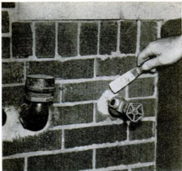
3. Above, old mortar around sill cock is removed and replaced with more permanent, epoxy mastic
