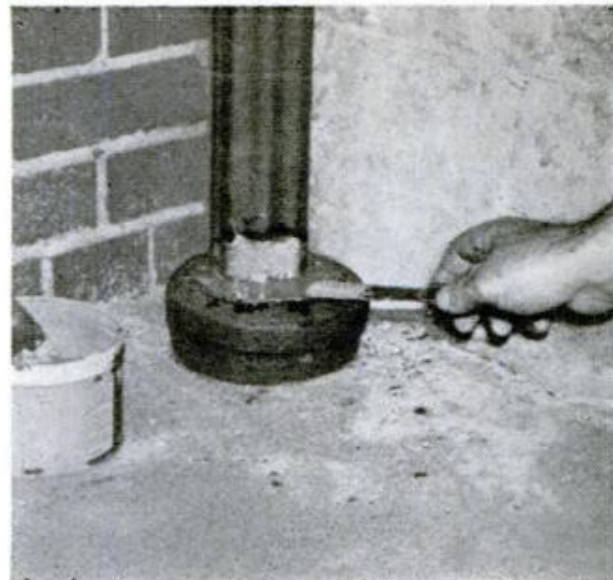
7. Loose downspout drain is calked with epoxy mastic, after wrapping with thin sheet plastic to keep it free for easy removal when a replacement is needed
