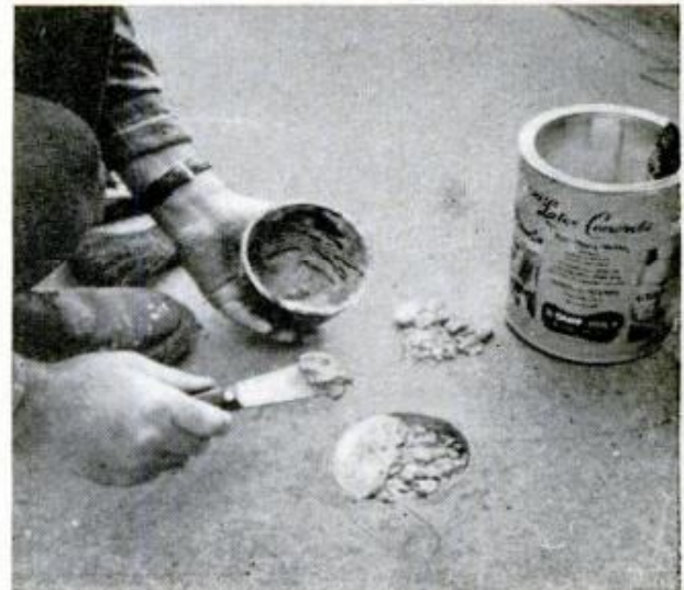
2. Hole left in concrete when fence was moved, is given rock filling topped with latex-mixed concrete
