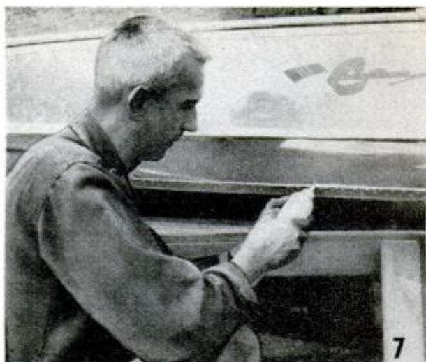
Above, leak in flat seam is stopped by applying sealing compound along lap edge and allowing capillary action of water in the joint to draw it into the void
