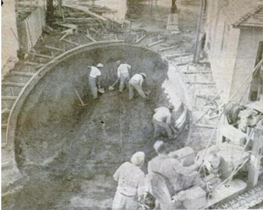
Once the excavation has been made work can move rapidly through several stages to the finishing touches. Note coping form
