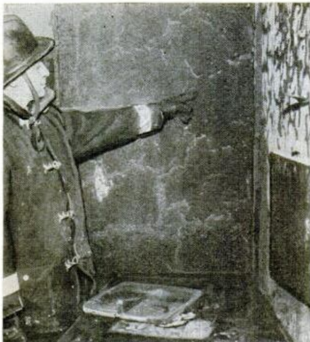
Only damage done to interior by fire was puffing of fire-retardant paint although furnishings were destroyed. Swelling, spongelike insulating puff is easily scraped off with putty knife and surface repainted
